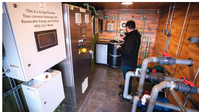
Control room for on-site AD facility. Photo courtesy of Impact Bioenergy
