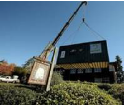
Impact BioEnergy's self-contained biodigester called HORSE is lifted by crane into place Tuesday at the Harbour Public House on Bainbridge Island. MEEGAN M. REID / KITSAP SUN
