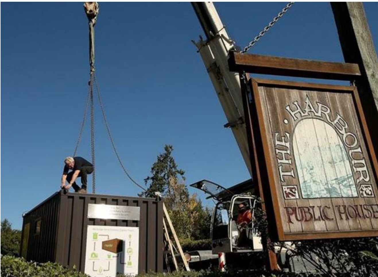
Impact BioEnergy's Jan Allen hooks the crane chains to the self-contained biodigester called HORSE before it is lifted and set into place Tuesday at the Harbour Public House on Bainbridge Island. MEEGAN M. REID / KITSAP SUN
